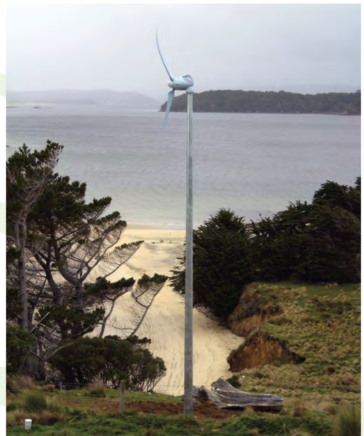
The wind turbine on Stewart Island, which is part of the renewable energy trial SIESA and Right House are carrying out.
