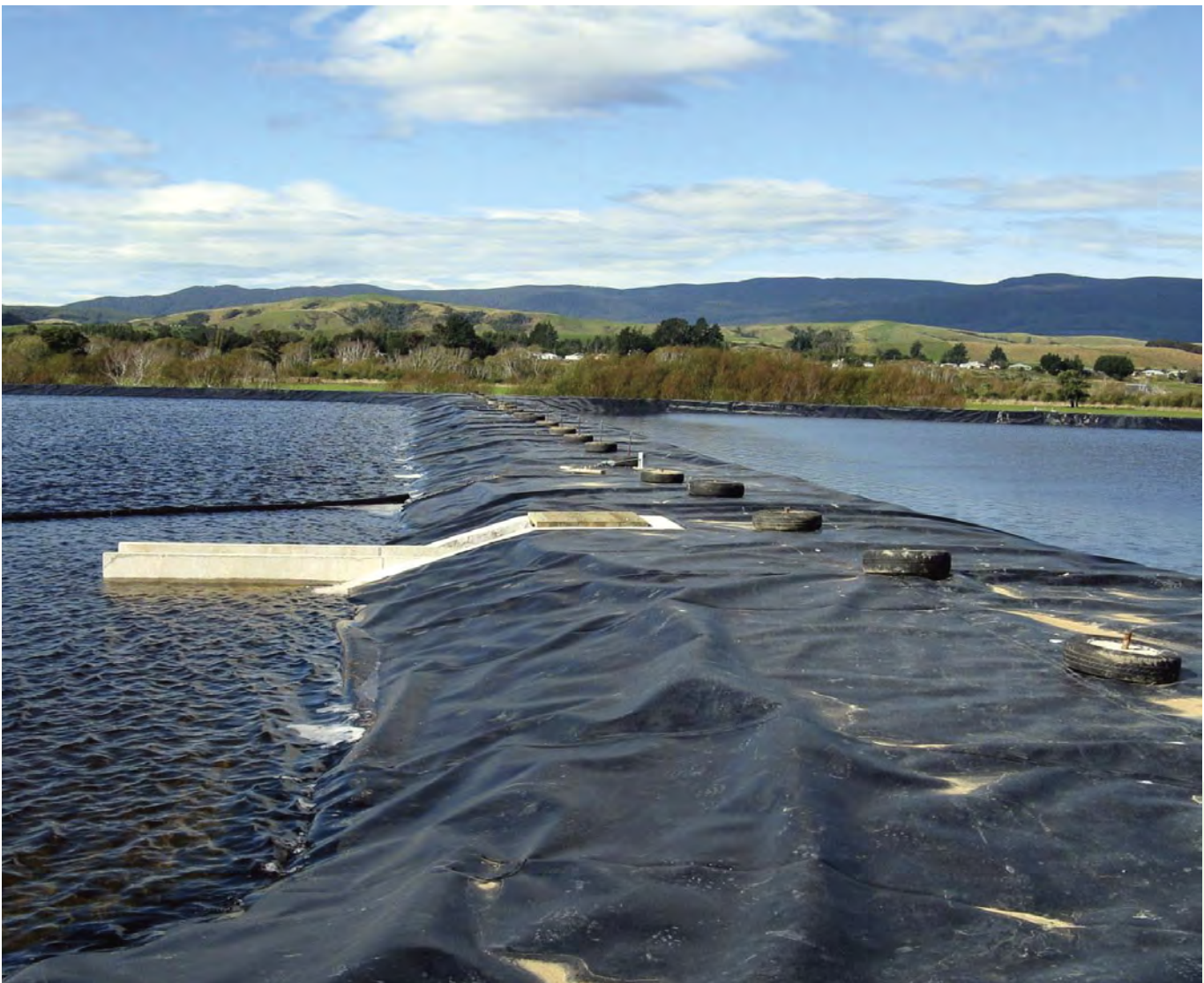
The ponds at the new Tuatapere sewerage scheme.
